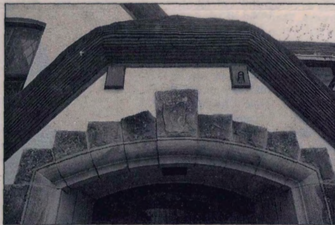
The cottage has an unusual thatch-effect, wood-shingle roof that is damaged and deteriorating. Fixing it would cost the congregation an estimated $75,000.
